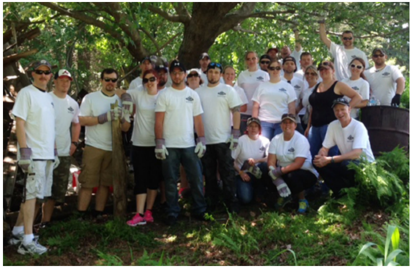
Texas Roadhouse Management volunteered and demolished the old wood shed on the Big Lake Trail.
